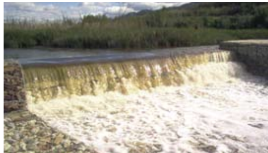
A retaining weir, built by Working for Wetlands, reduces erosion of a montane stream during summer flooding.
