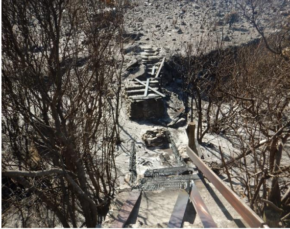
Fig 1 – Fire damaged Attwel bridge
