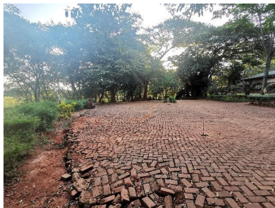
Fig 2: Paving area that needs to be reconstructed barrel roof
