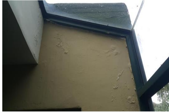
Fig.4. Paint bubbling caused by leaking concrete slab
