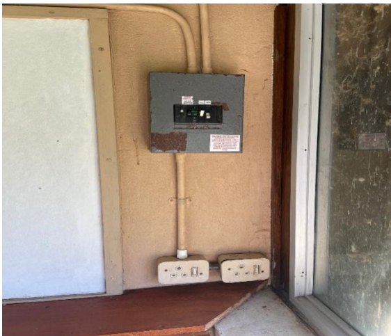
Fig 5. Existing distribution board
