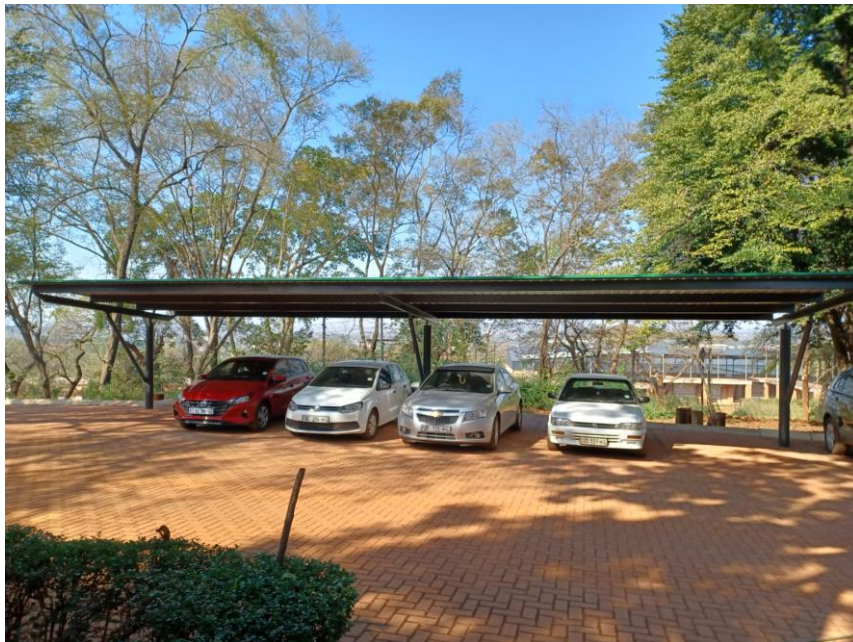
Typical Covered Parking to be installed.
