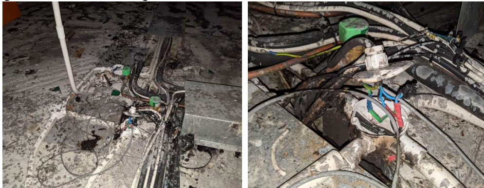
Figure 2-6: Other cable damages
