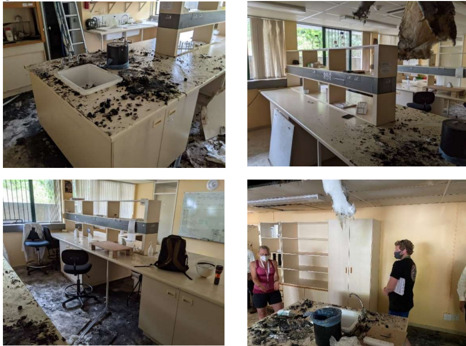
Figure 2-13: Joinery work damages
