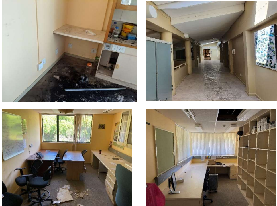
Figure 2-12: Floor covering damages
