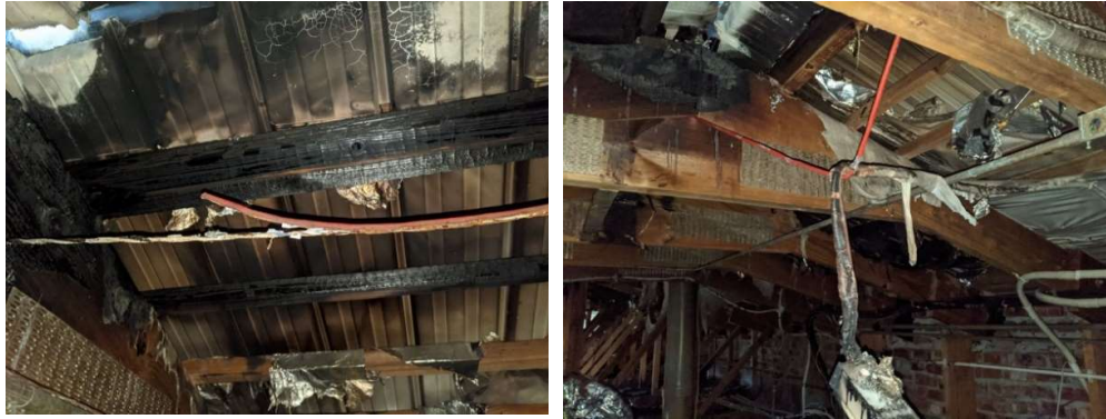
Figure 2-5: Main supply cable
