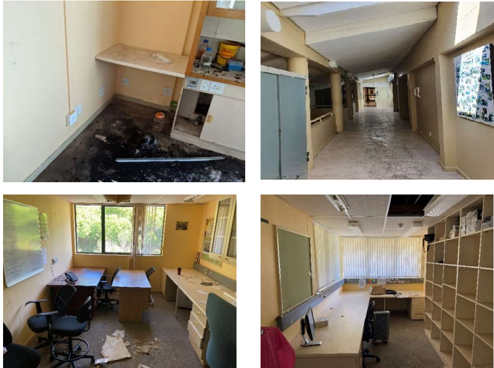
Figure 2-12: Floor covering damages
