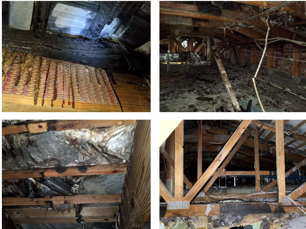
Figure 2-1: Roof truss damages
