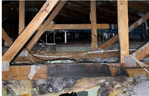
Figure 2-10: Fire detection damages
