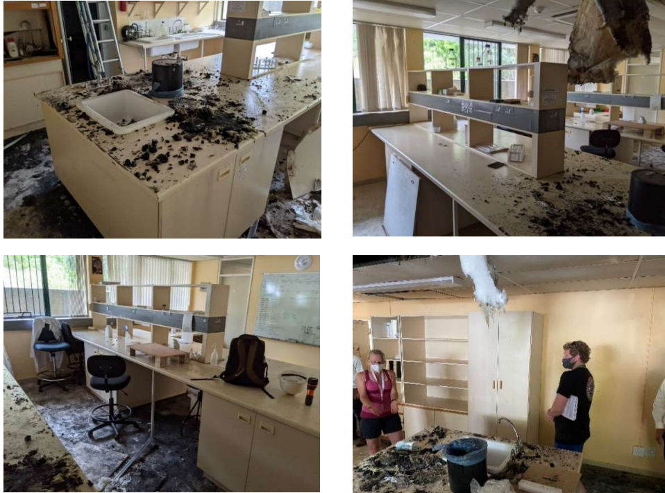
Figure 2-13: Joinery work damages
