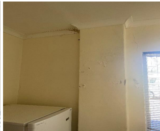
Fig 6. Internal damp wall and column
