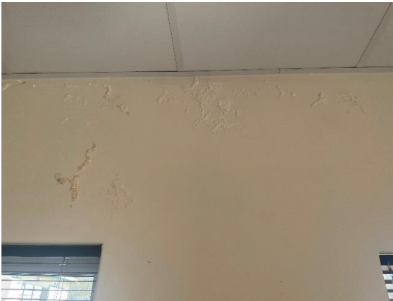
Fig 5. Internal damp wall
