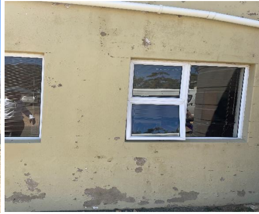
Fig 4. External damp wall
