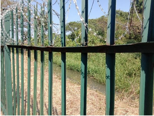
Fig 2: Palisade fence that needs painting maintenance
