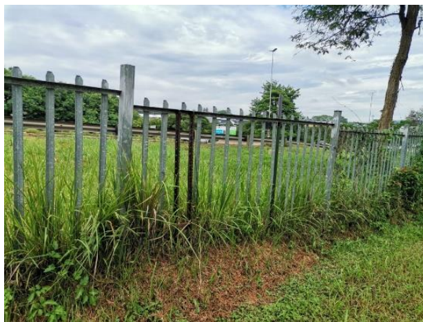
Fig 4: Damaged palisade fence that need replacement.
