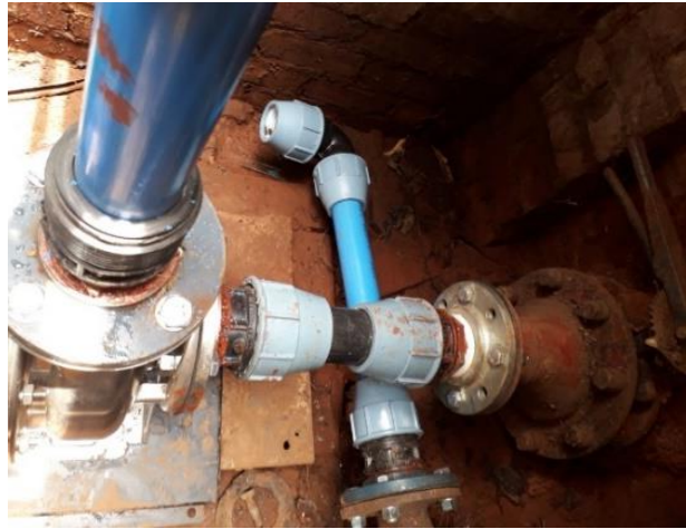
Waterfall Circulation Pump pipes & Plumbing
