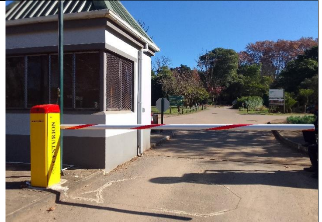
Fig.2: Existing Exit Boom gate with ground loop detectors
