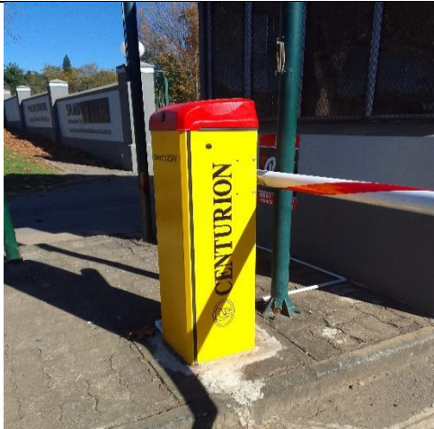
Fig.3: Existing centurion boom gate system box
