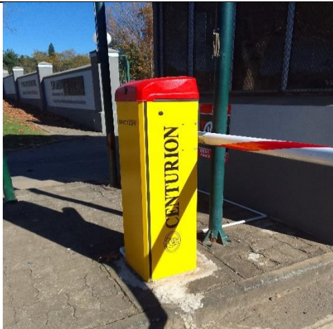
Fig.3: Existing centurion boom gate system box
