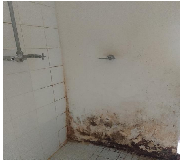
Fig.2: Wall needing tiles
