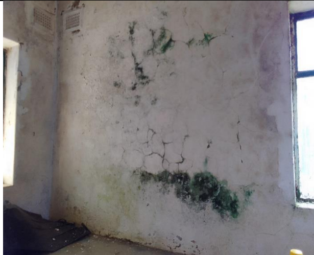
Fig.3: Interior walls to repair
