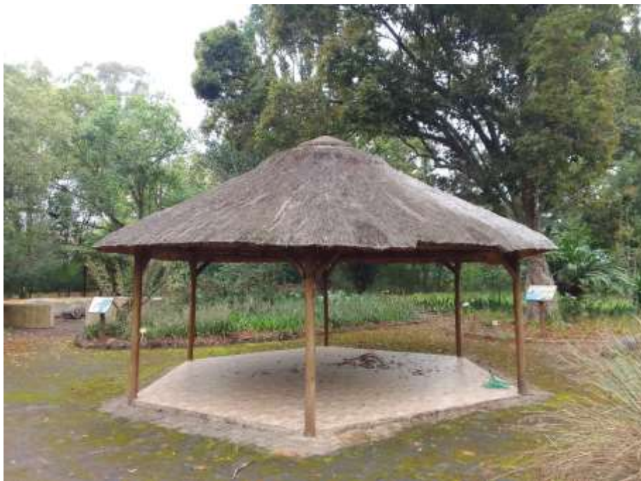
A thatched Lapa requiring repairs
