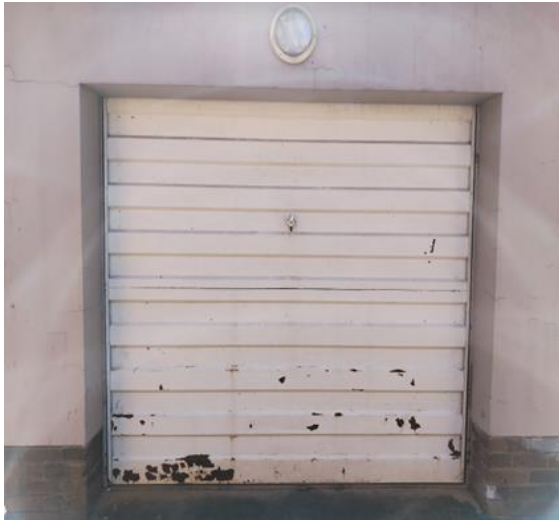
Fig.1: Existing Garage door that needs to be replaced with automated one.
