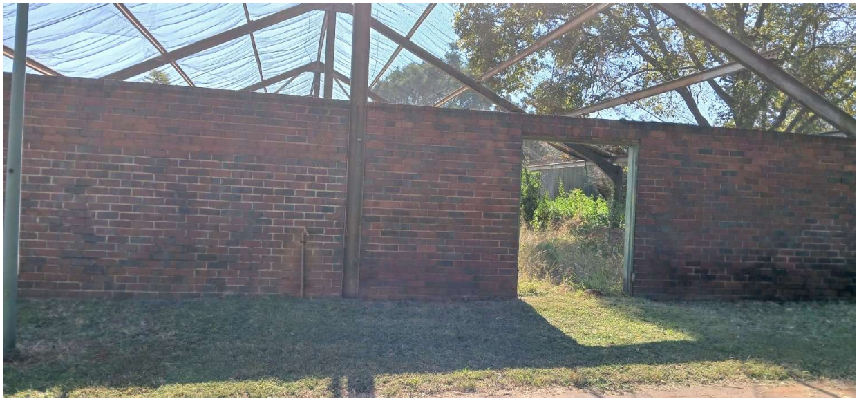
Figure 6: Irrigation system needs to be installed
