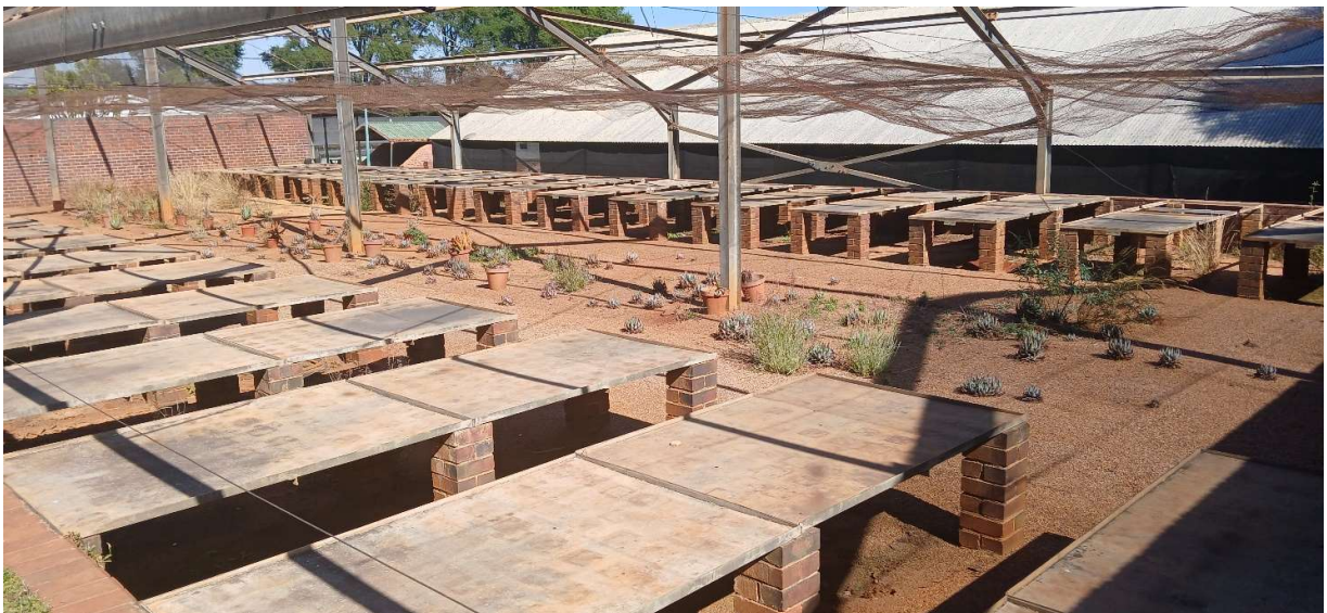
Figure 2: Nursery asbestos tables that need to be replaced with galvanised steel
