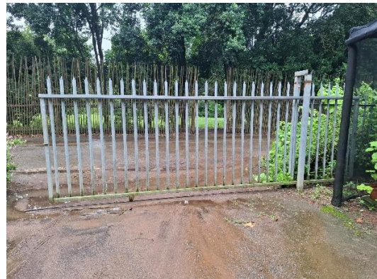
Fig.4: Existing gate that requires gate motor and inbound and outbound keypads
