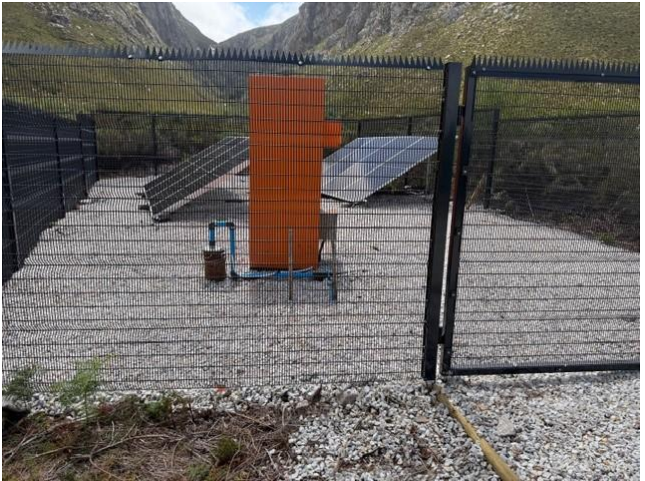
Fig.1. Typical example of completed installation (Project Solar PV Plant design will vary)
