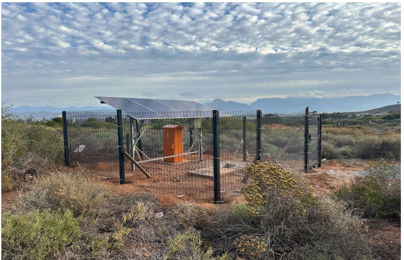
Fig.2. Typical example of completed installation (Project Solar PV Plant design will vary)
