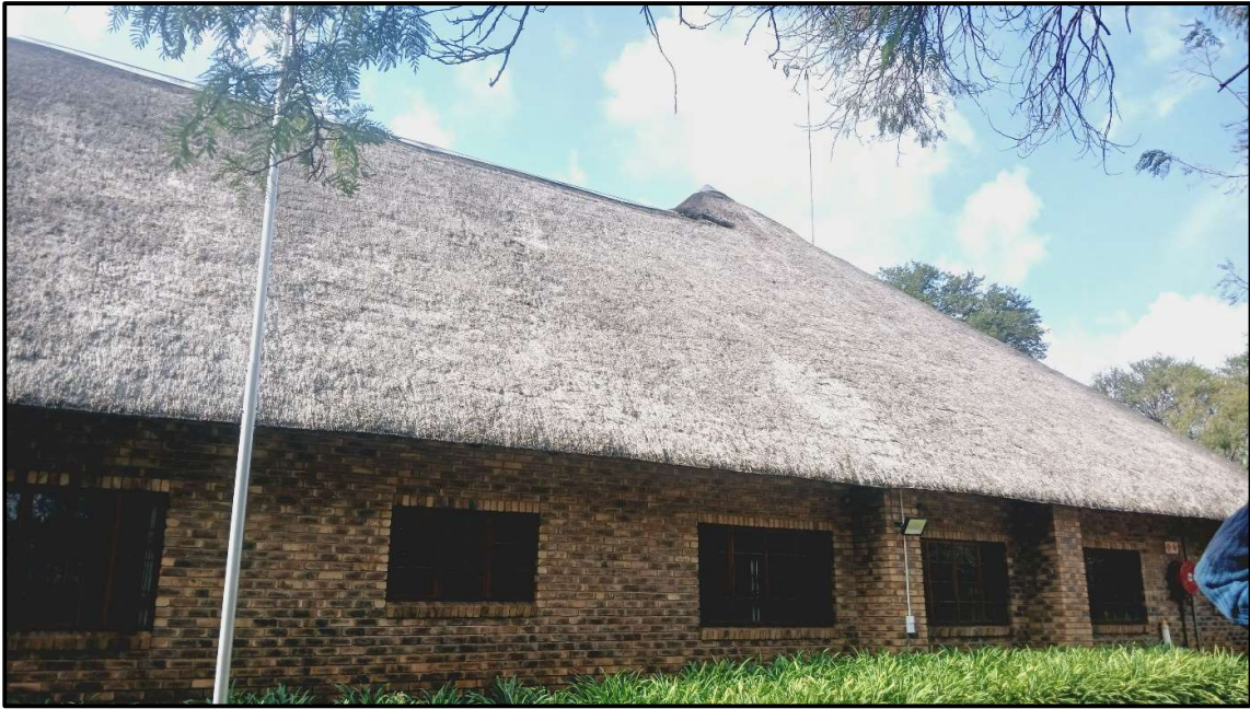
Figure 1: Side of the Thatch roof Education Centre that needs repairs
