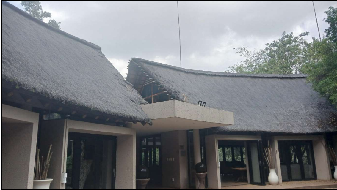
Figure 3: Thatch roof that needs repairs at Milkplum Café
