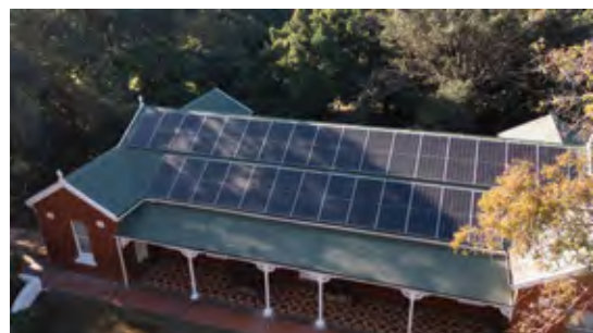
Solar PVs installed at the KwaZulu-Natal Herbarium, Durban, KwaZulu-Natal.
